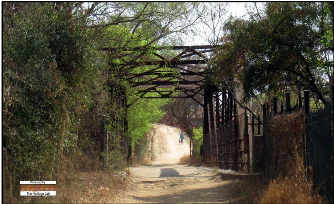
Figure 8. Old single lane metal truss road bridge north of the project area
